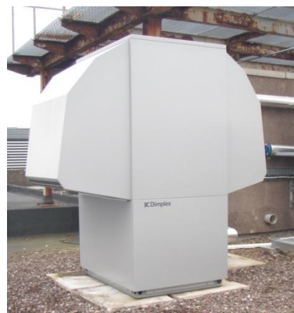
Fig. 5 AIR SOURCE HEAT PUMP ON ROOF OF ZERO2020 BUILDING
