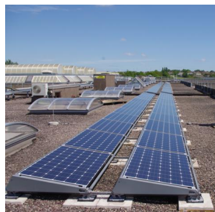
Fig. 7 INSTALLED PV ARRAY ON ROOF OF EXISTING BUILDING
