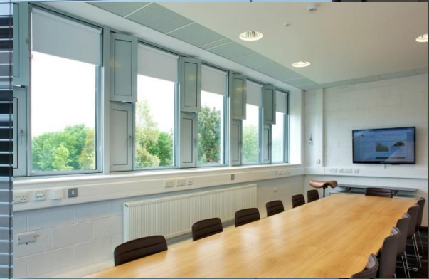
manual & automated purpose provided ventilation openings with insulated doors
