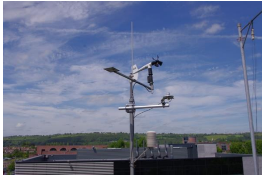
Figure 3.2: Picture of weather station located on the roof of the building
